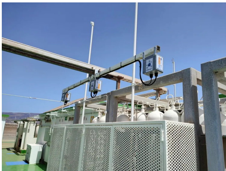
Figure 1: Typical hydrogen leak detection sensor installation in storage tanks.
